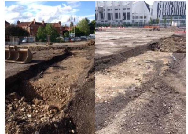
Previous site condition with the tarmac being stripped prior to groundwork's. No vegetation has existed on this site for a number of years.
