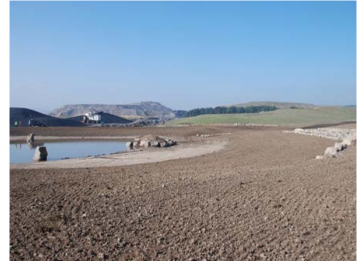
Soil forming works and land shaping complete ready for planting and seeding.
