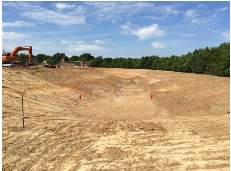
Photo: Attenuation pond to manage storm water
