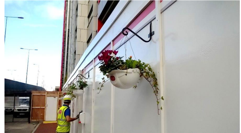
Rathbone Phase 3 project: Sisk hard hats planted with pollinating plants and hung on site hoarding.
