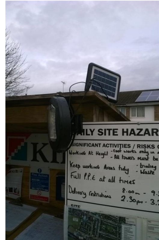
Solar powered light used on site
