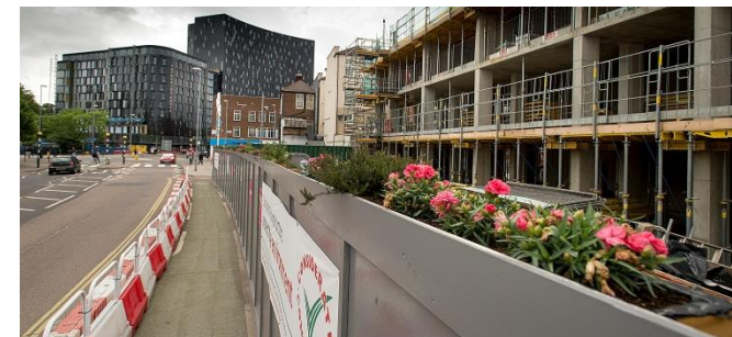
Top : Aerial view of site. Pink: Number One Portsmouth, Yellow: bus route, Blue: Portsmouth & Southsea Train Station, Green: adjacent town centre. Bottom : Taking advantage of available space with Meadow Wildflower and Lowland Heath planters on top of our hoarding
