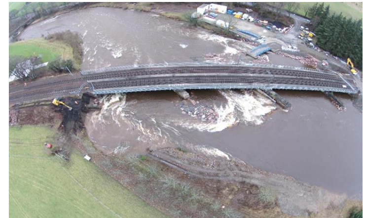
Photo Description: Lamington Viaduct, January 2016. Prior to construction works commencing. Scour of the embankment evident
