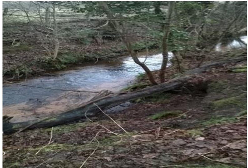
Photo: Scoured Embankment before the works started
