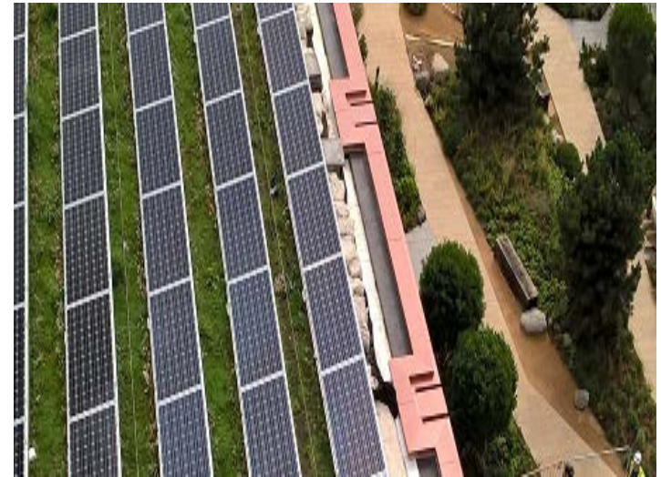
View from top roof, showing roof 2 green roof an PV array, also showing a small section of podium roof.
