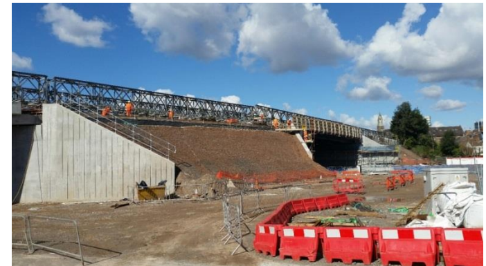
Top – Layout showing embankments where wildflower seeds sown. Below – Photo showing embankments during construction phase.
