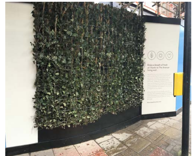
Photo Description: APU installed as part of the hoarding design
