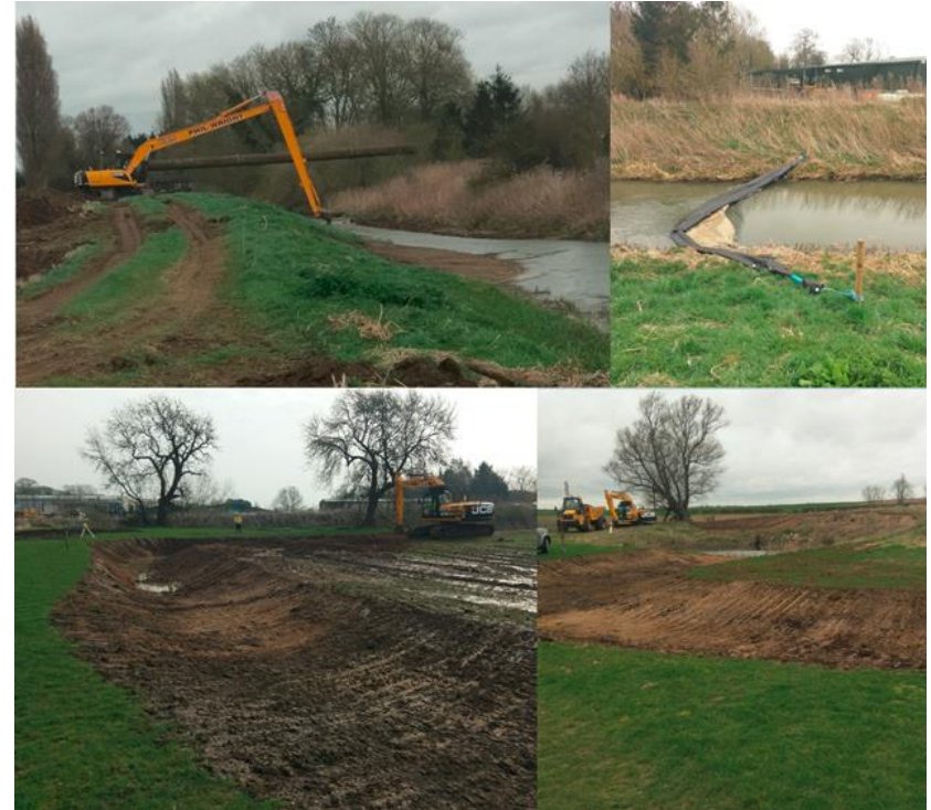
Photo Description: The construction Process and methods used, including top right silt capture in the main river
