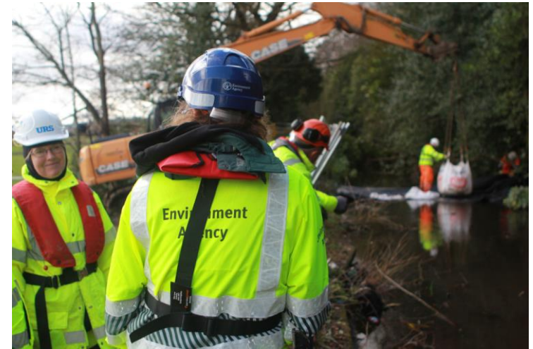
Photo Description: River diversion works in progress ahead of crayfish rescue and translocation
