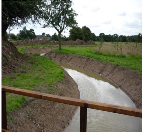
The right hand sides shows the new orchard area, the left hand side earth spoil will be landscaped to provide additional flood protection to the house.
