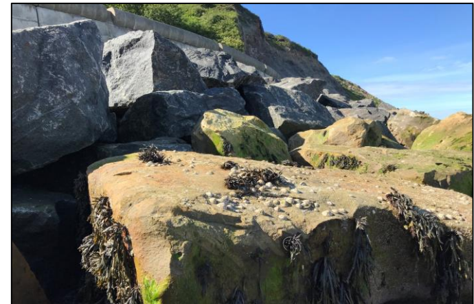
Natural existing boulders placed at the toe of the new structure to aid colonisation of granite boulders
