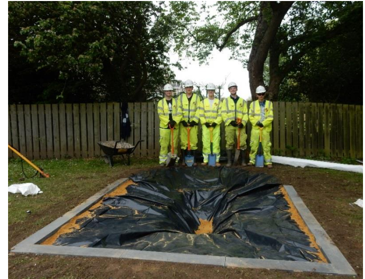
Construction of dipping pond at All Saints School by Morpeth Northern Bypass engineers and apprentices
