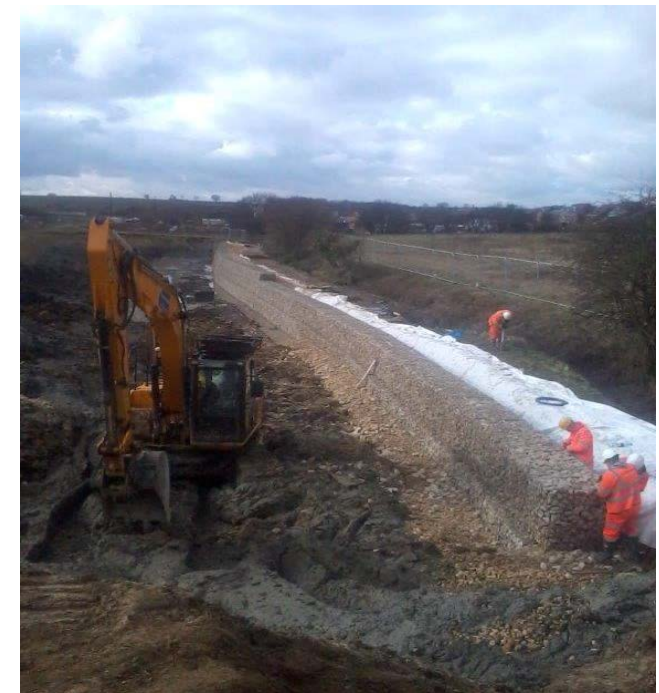
The picture shows work getting underway at Linear Park, which runs from one side of the development to the other and will continue to be developed as further phases of land are built upon by Kier Living Eastern.
