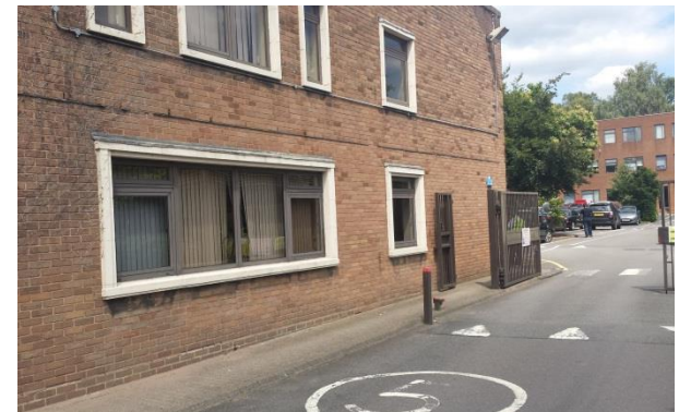
Photo Description: Entrance to Interserve offices. Bee hive is in the cavity above the large window.
