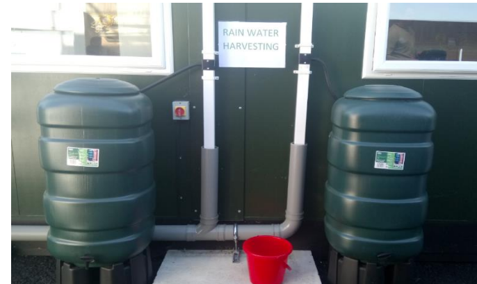
Photo Description: Rainwater harvesting used for watering the vegetable garden.
