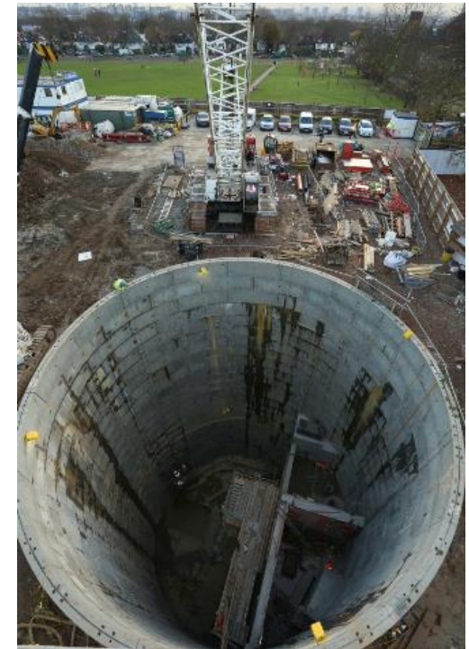
Above: The overflow tank, a key part of the flood alleviation scheme in construction in Tiverton Green. The community orchard and wildflowers were planted where the crane and car parking is located.
