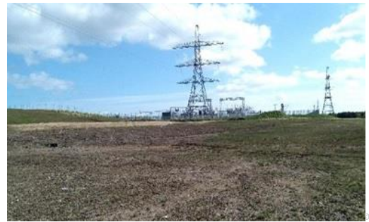
Thurso South Substation, SSEN
