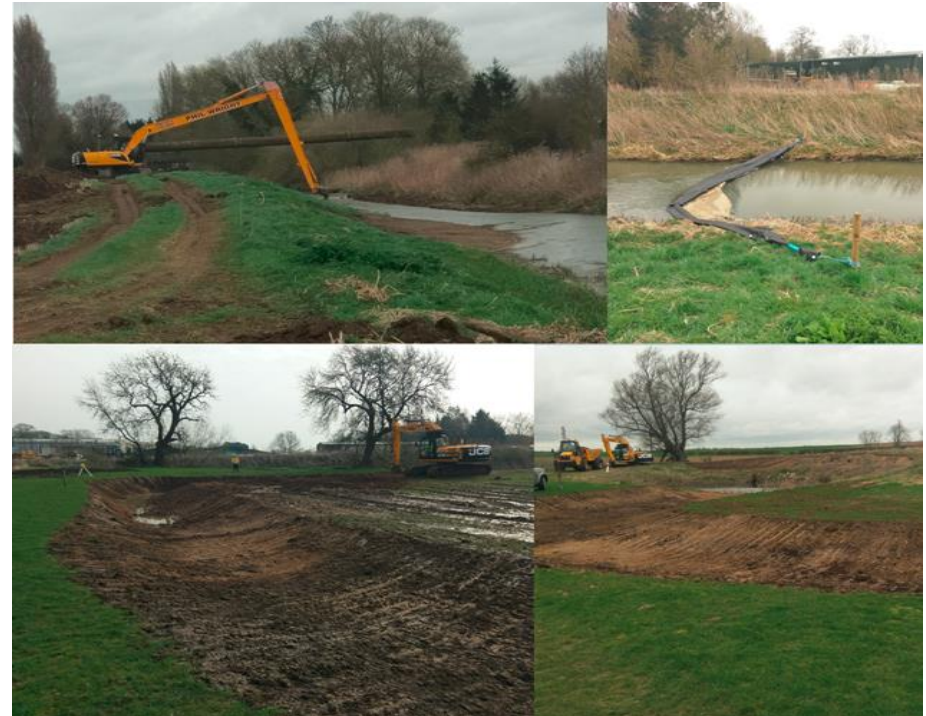
Photo Description: The construction Process and methods used, including top right silt capture in the main river
