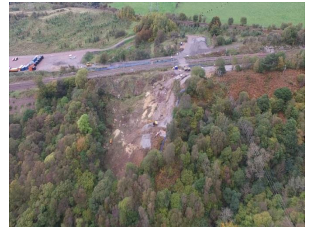
Slope prior to intervention works, West Coast Mainline running left to right through photo:
