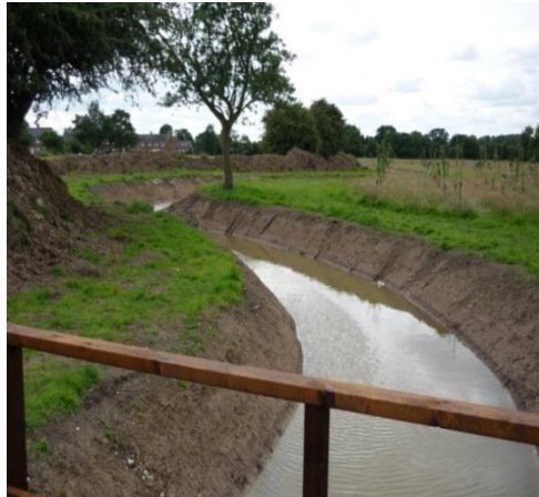
The scheme in progress the right hand side earth spoil will be landscaped to provide additional flood protection to the house.
