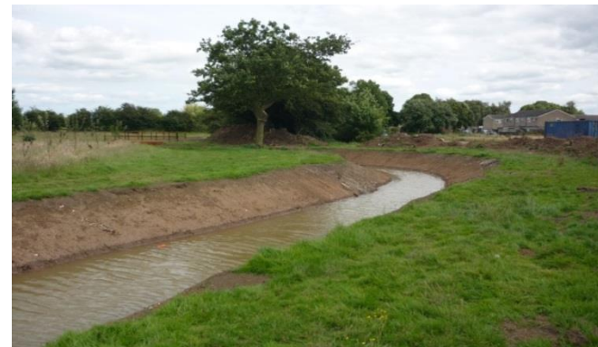
Daylighting of the culvert with a meandering bend around the existing trees
