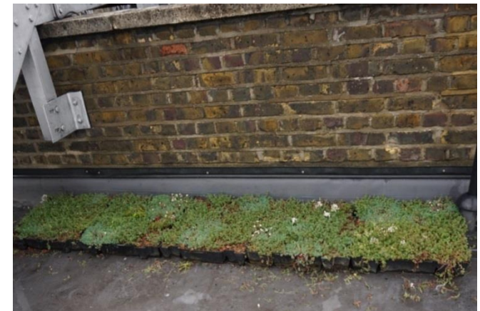
Sedum pods in situ on service roof at 71 Broadwick Street, Carnaby
