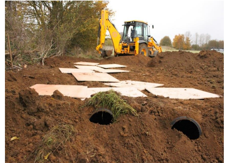
During the creation of the artificial badger sett at Westhill the plywood boards, which would form the nesting chamber, were laid out on the ground.
