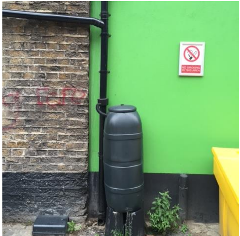
Photo: Rainwater harvesting
