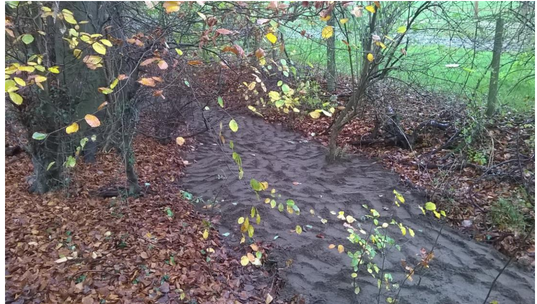
Photograph taken immediately after the reinstatement of the gully in the ancient woodland.
