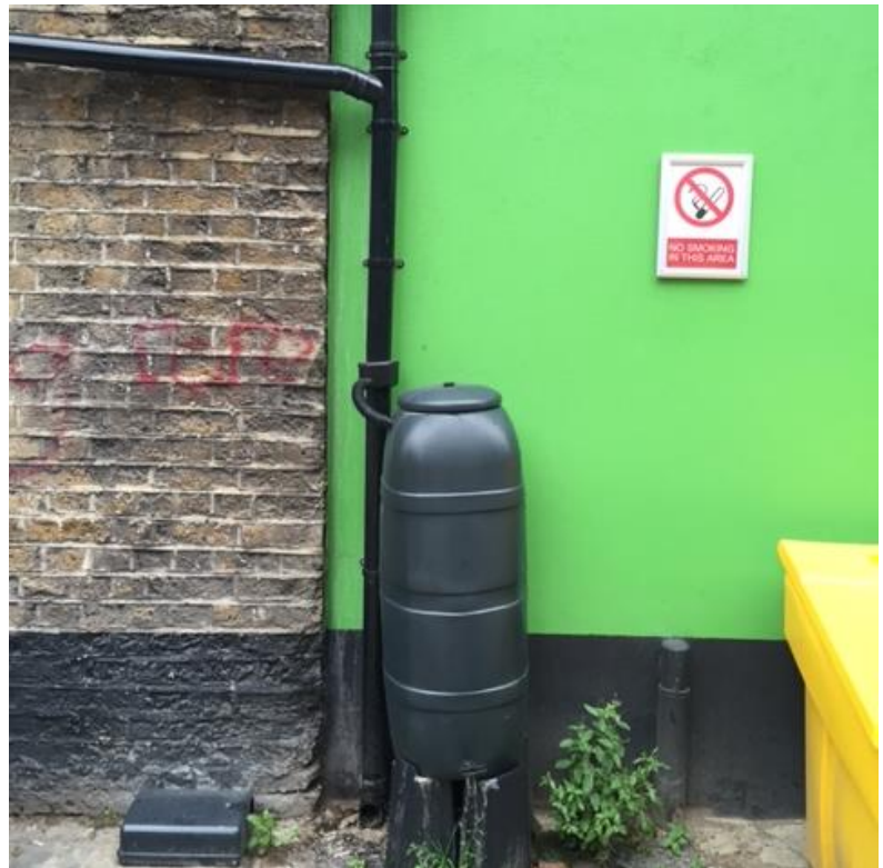
Photo: Rainwater harvesting
