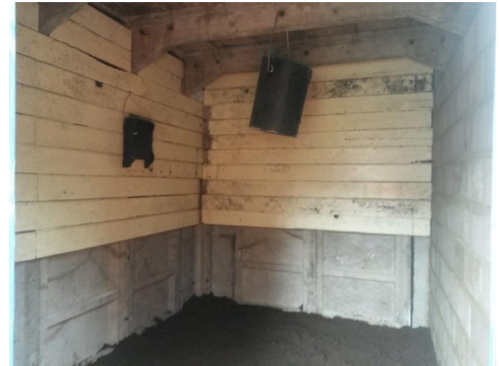
View into the enhanced relay room from the main door. To the right is the breeze block wall with gaps for bats to roost in. Front and to the left is the wooden panelling with space underneath to enable monitoring. Two bat boxes included in the building, one suspended from the concrete beam and another mounted on the wall. Soil on the floor improves temperature and humidity.
