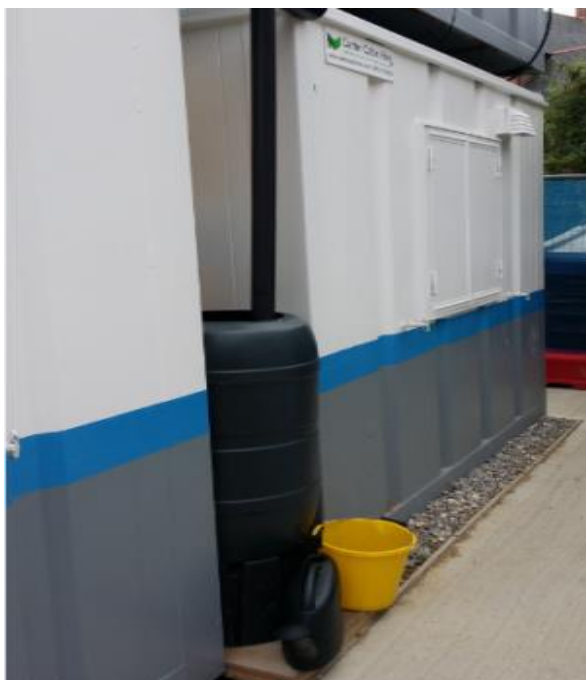
Photo: Rainwater Harvesting
