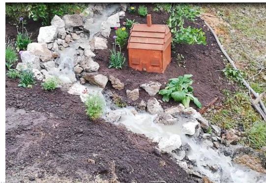
Spooner Row waterfall and pond filter in construction and end result – J England
