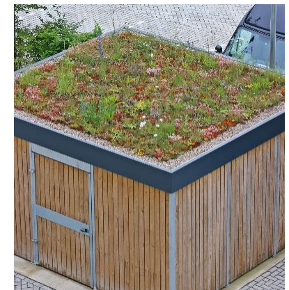
Green roof planting on store buildings
