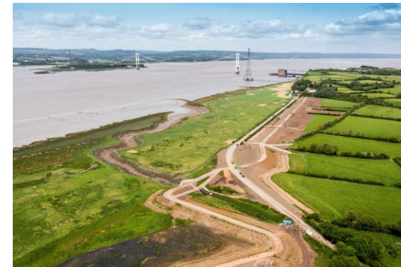
Earth embankment construction with outfall structure in the foreground which we raised the height of.
