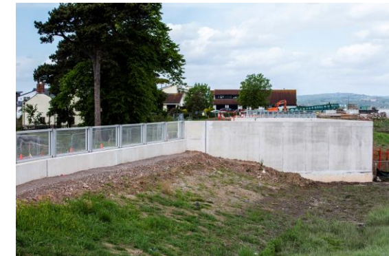
Glass panels in the flood defence walls at New Passage with an outfall structure which has been increased in height.....
