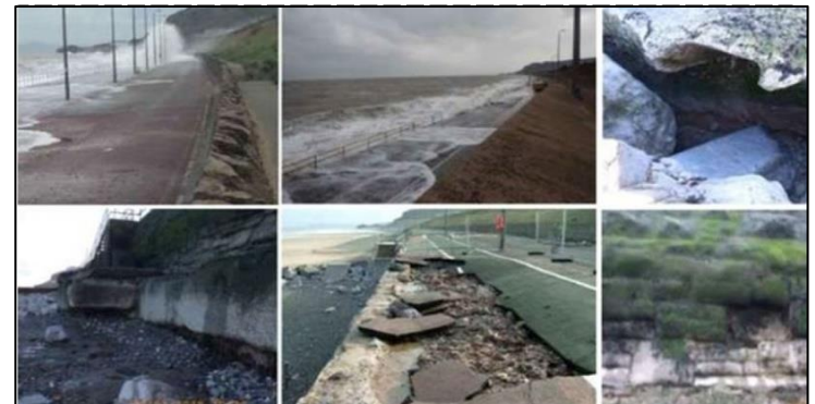
Examples of recent storm damage - Conwy County Borough Council
