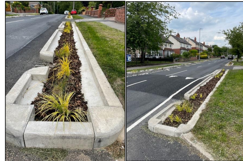
Rains gardens have been planted with a combination of shrubs, grasses and a lowland meadow mix.
