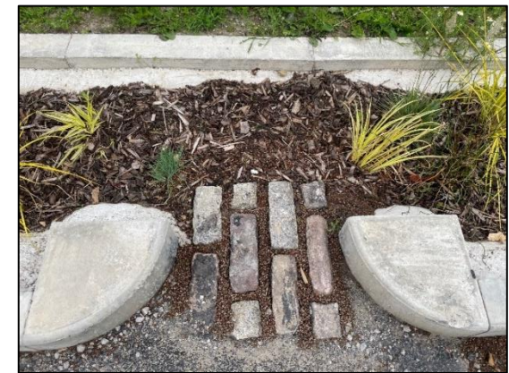
The dissipation blocks at the rain garden inlets utilised cobblestones extracted from the initial road excavations
