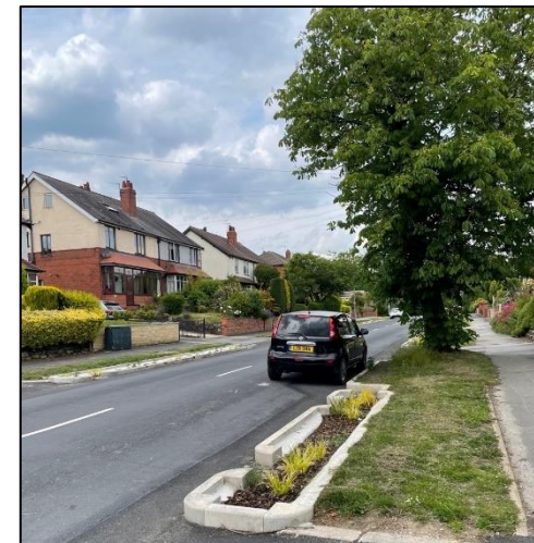
Rain garden installed around existing trees, preventing root damage and in keeping with the sustainability drive of the scheme.
