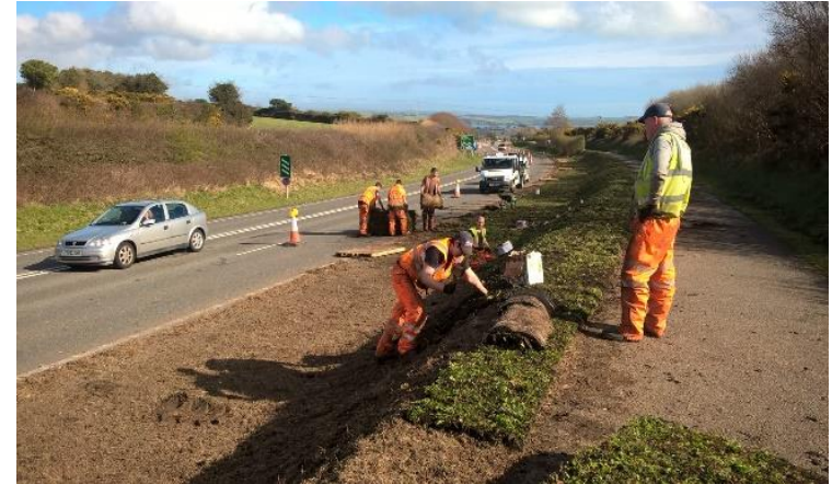
St Austell A391: Following a turf strip by mechanical means avoiding glyphosate, wildflower turf is laid to the highway verges (Photo By Cormac)
