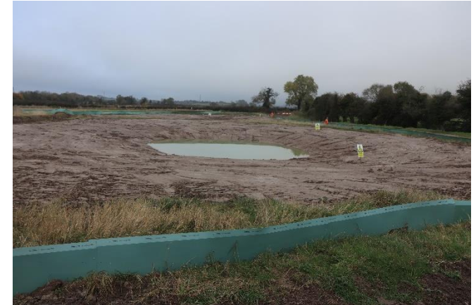
Construction of newt pond with newt fencing so that they could be relocated during construction activities. The newt fencing is then removed and replaced with stockproof fencing to protect them from cattle.
