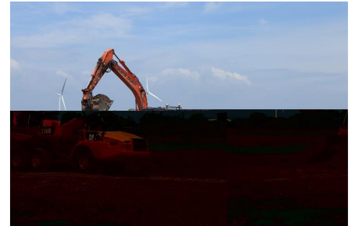
Cut and fill to reprofile areas, with all excess materials generated used elsewhere on site for construction of embankments.
