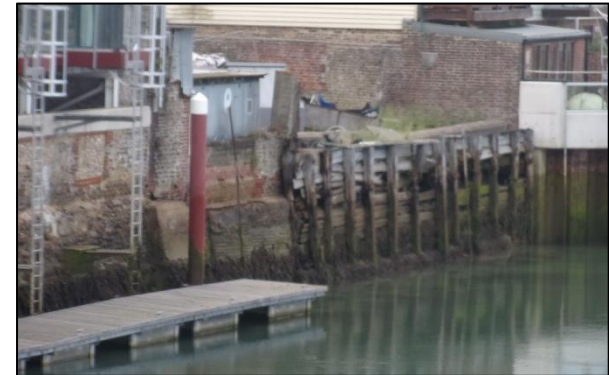
Description: The site prior to a new flood defence. Image courtesy of Mackley.
