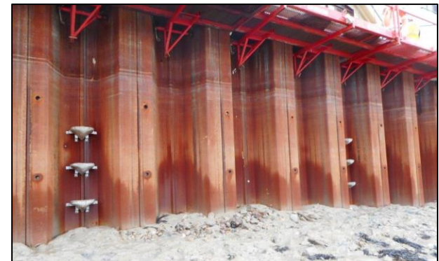
Description: The site following installation of new sheet piling and Vertipools. Image courtesy of Mackley.
