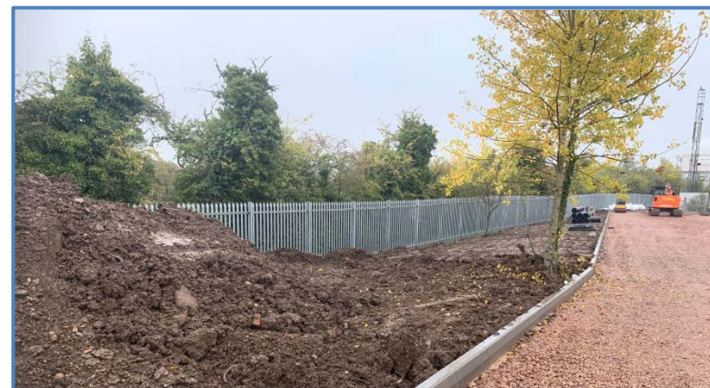
Top soil being stored ready for spreading. Re using the top soil is not only a cost saving it limits the risk of importing unknown species and reduces lorry movements.
