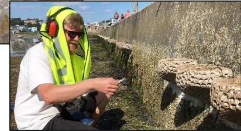
Top: a rockpool being made with the bubblewrap lining the mould. Bottom: the rockpools being installed at Sandbanks, Poole Harbour by Artecology.
