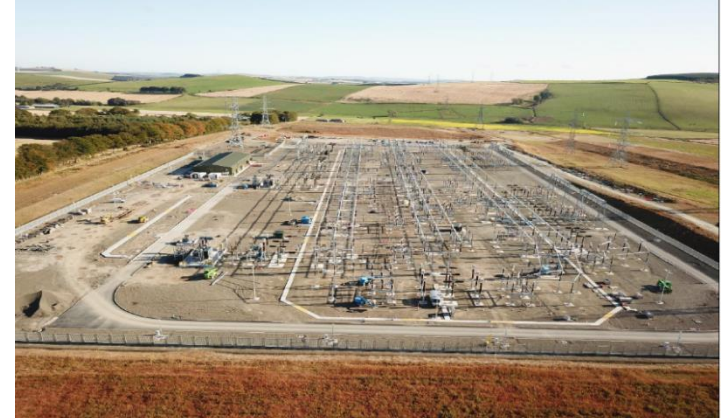
Completed construction of Rothienorman AIS (Air Insulated Switchgear) Substation (image credit: Siemens+BAM)
