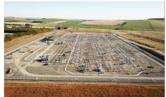
Completed construction of Rothienorman AIS (Air Insulated Switchgear) Substation (image credit: Siemens+BAM)
