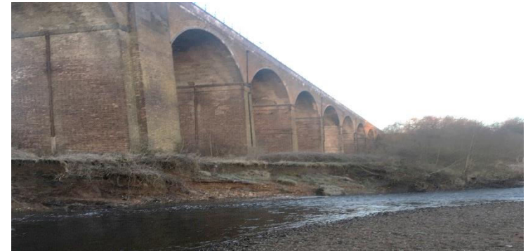
Heavy Scour to the Western Bank:
