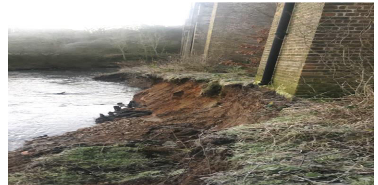
Scour exposing the foundations of the viaduct:
