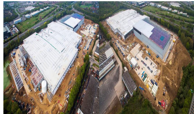
The Crown Packaging facility in development on the site – retained areas of open mosaic habitat can be seen along with new areas of habitat works
